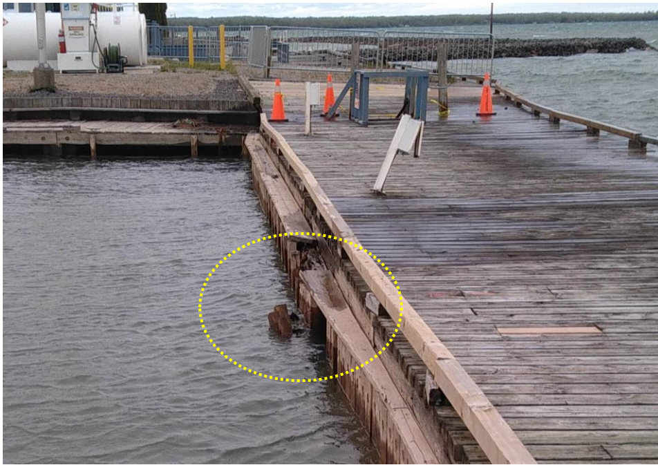
Figure 1: Dislodged vertical timbers inside east basin.
