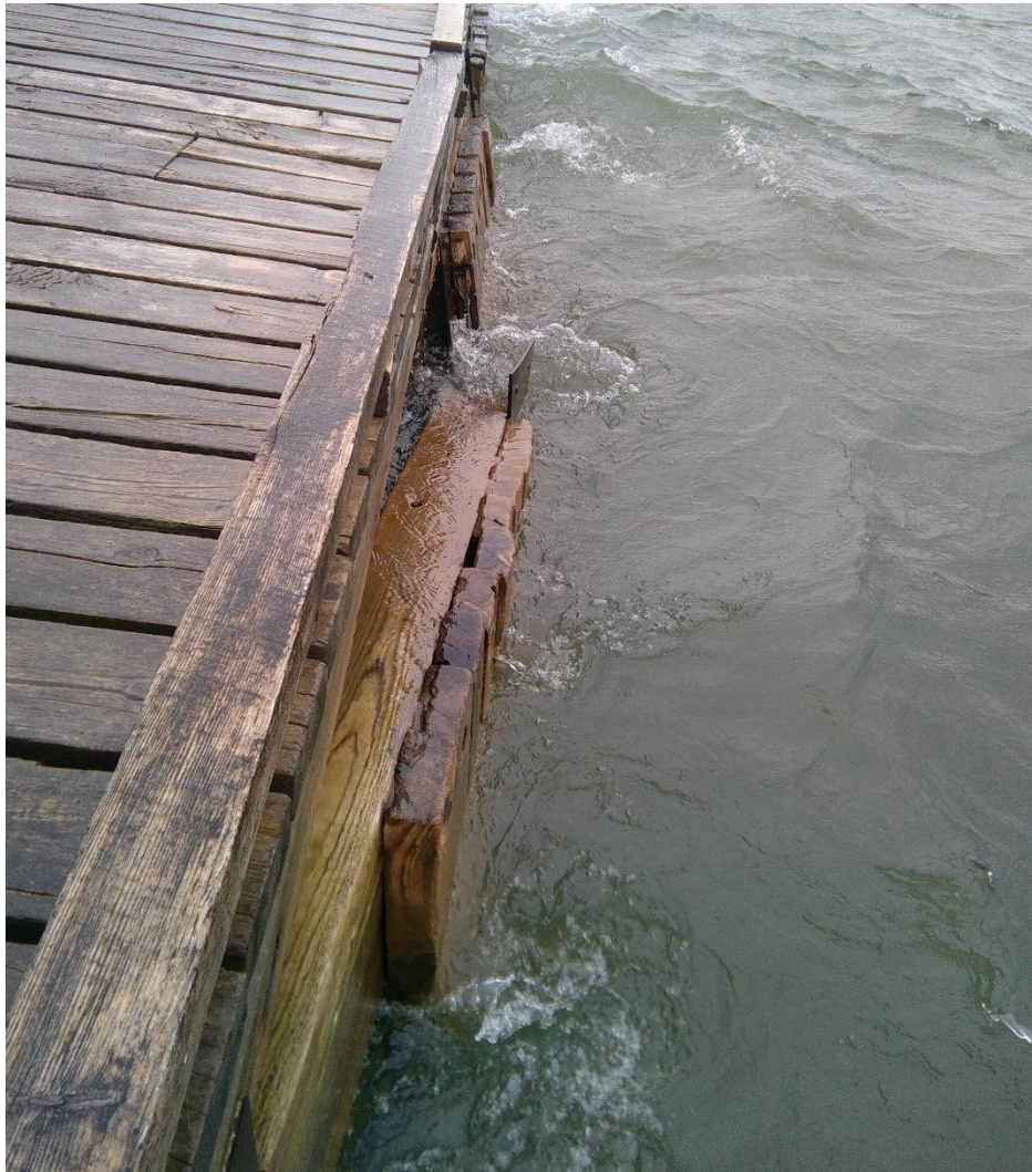
Figure 3: Horizontal dock framing member separated from crib, north side.
