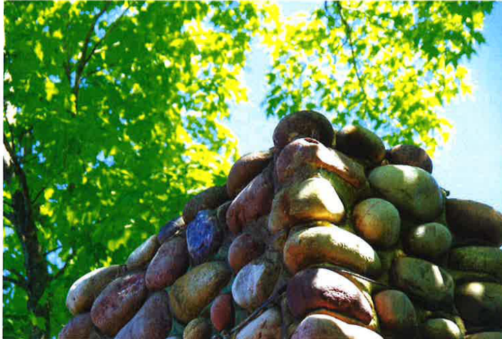
Photo 9: Top of stone chimney. Note lack of rain cap and steel cable wrap.
