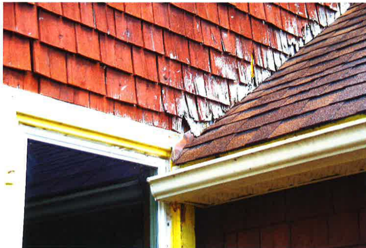
Photo 10: Roof wall interface at rear of south addition. Note siding deteriorated.
