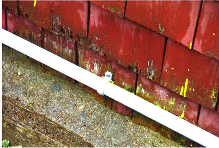
Photo 11: Typical condition of siding near foundation level.
